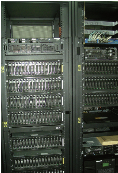
Each rack has one HELIOS Server and attached RAID system.
